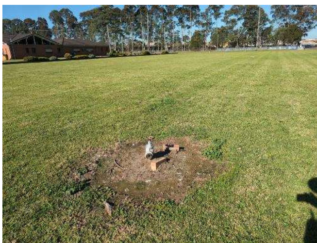
Figure 20. Irrigation tap identified in western project area.
